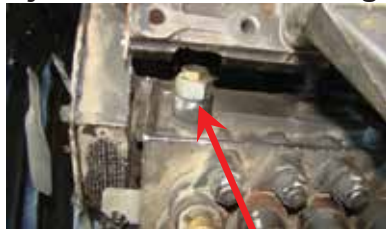
Figure 56 Return Line From the P-7100 Pump
