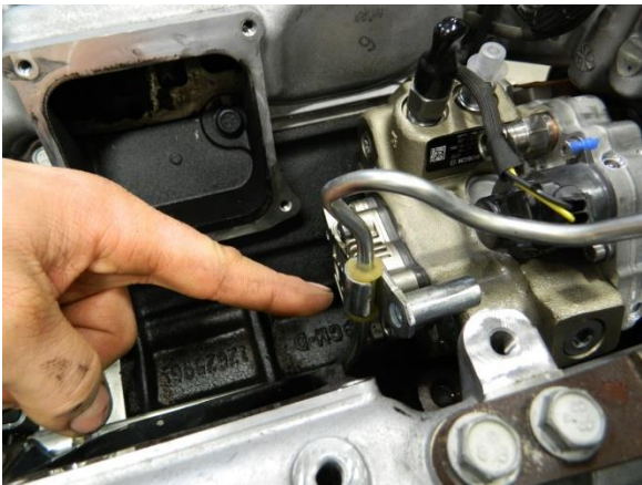
Fig. 14: Carefully remove high pressure line bracket
